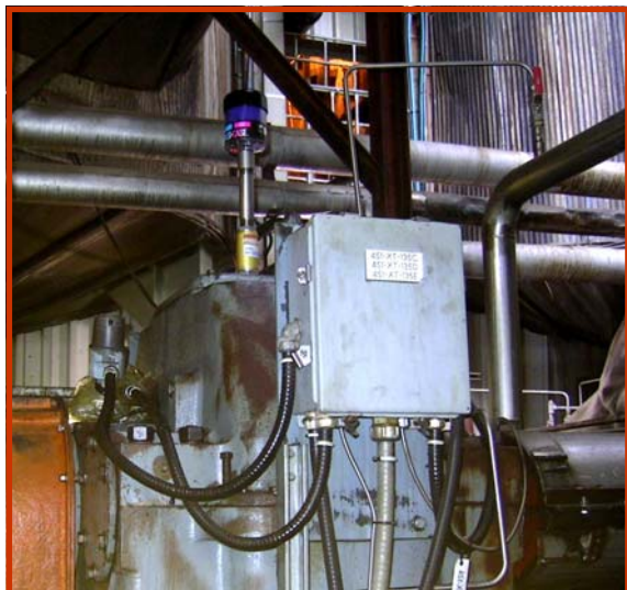
KILN DRIVE SPEED REDUCER
